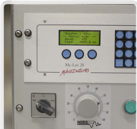
NC control panel
